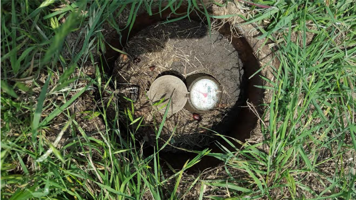
Photo 10 – Cycle 17 Meter at 315 Roseburd Ln (replace meter box with SAWS standard; clean out excessive dirt/debris in meter box):
