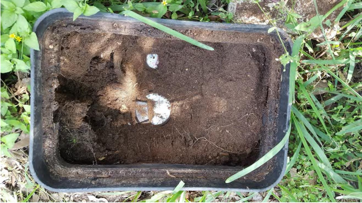
Photo 6 – Cycle 6 Meter at 145 Timbercreek Rd (2 meters in same box): Replace with 1 larger meter box.
