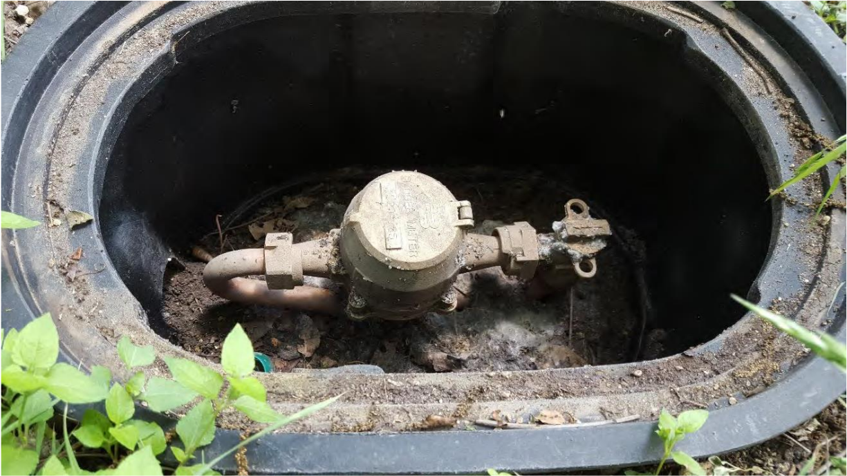
Photo 12 – Cycle 17 Meter at 1333 Stonewll Street (yoke required to raise meter closer to grade):
