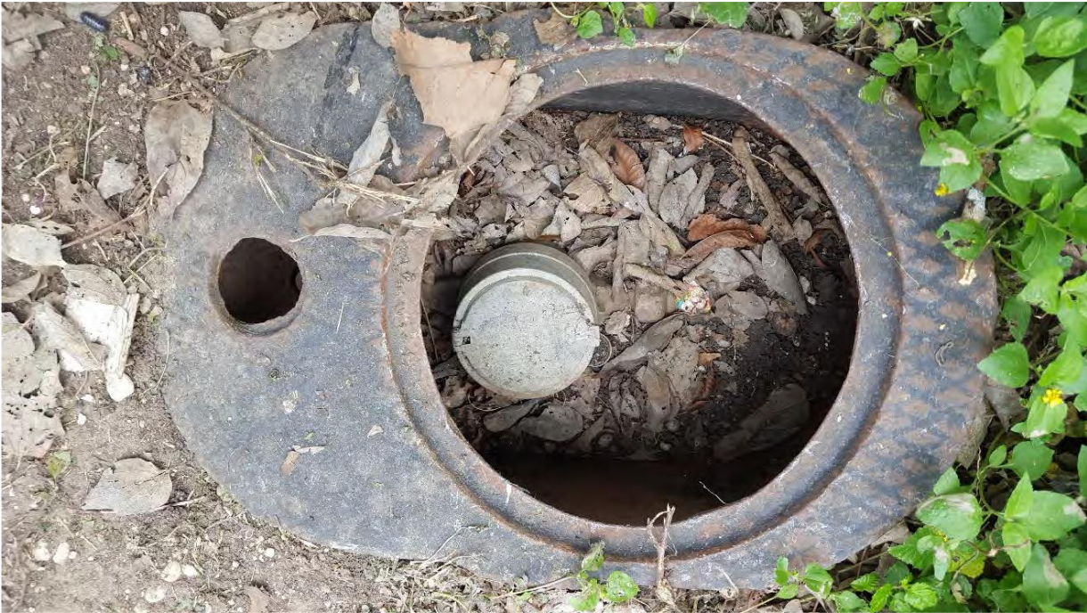
Photo 11 – Cycle 17 Meter at 330 Sims Ave (replace meter box due to poor condition and to faciitate access; clean out excessive dirt/debris in meter box):
