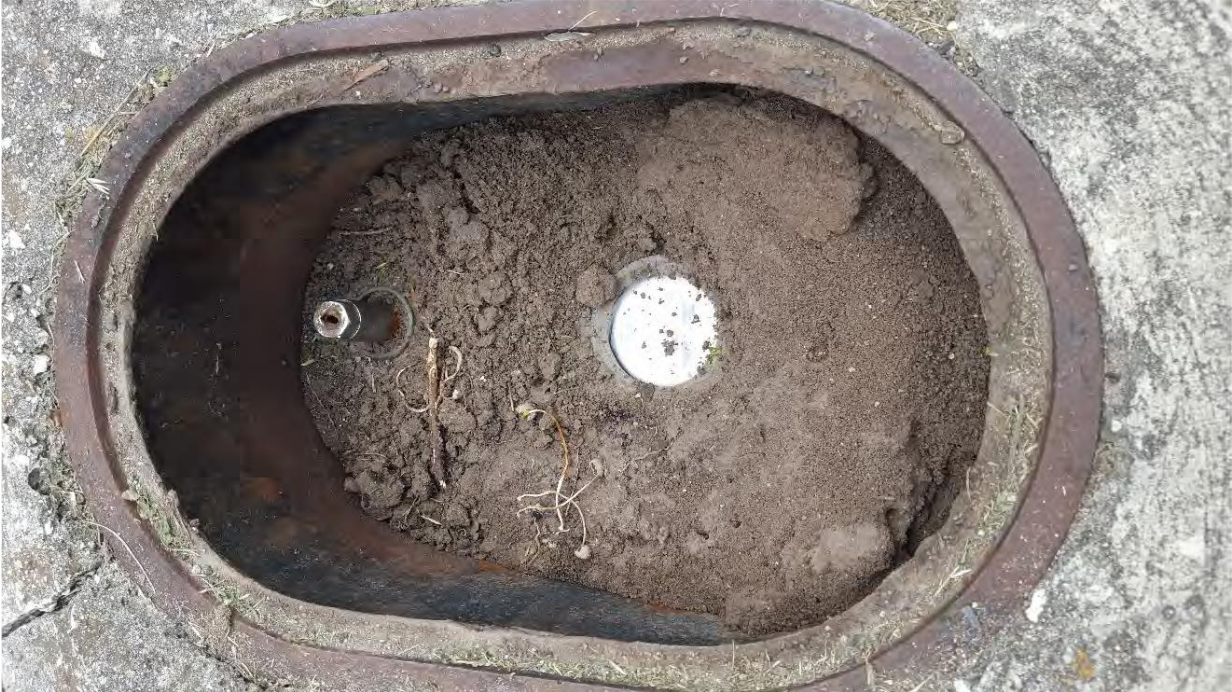
Photo 5 – Cycle 6 Meter at 8327 Robin Hill Dr (clean out excessive dirt/debris in meter box; verify if curb stop valve is functional):
