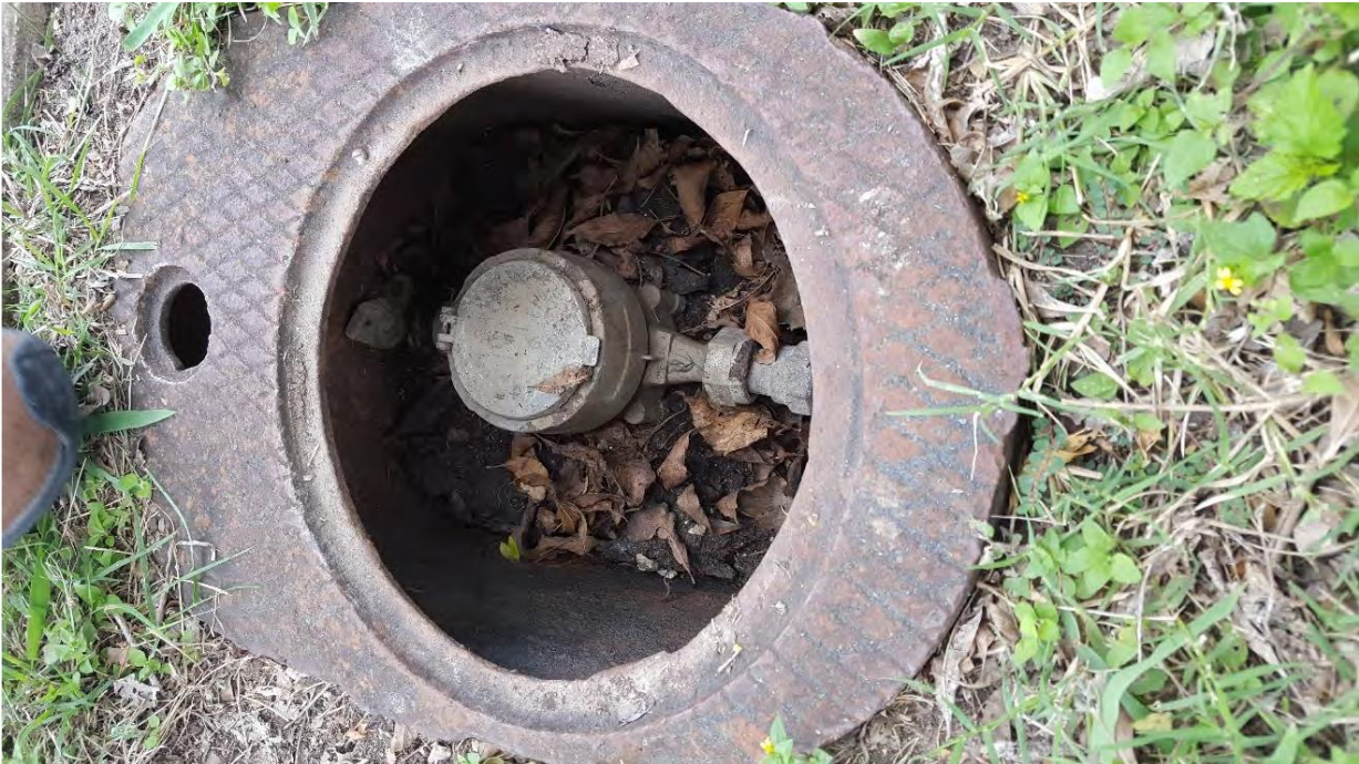
Photo 9 – Cycle 17 Meter at 211 Hoover Ave. (replace meter box with SAWS standard to facilitate meter replacement and access to curb stop):
