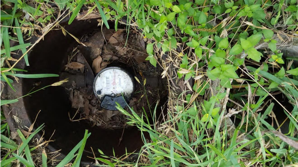
Photo 13 – Cycle 17 Meter at 478 E Hutchins Place (replace meter box with SAWS standard; clean out excessive dirt/debris in meter box):
