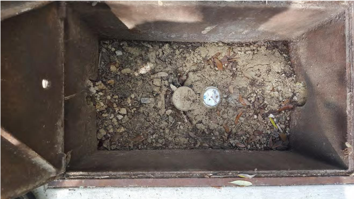
Photo 3 – Cycle 6 Meter at 2703 Marlborough Dr. (clean out excessive dirt/debris in meter vault; add yoke to raise meter to grade):
