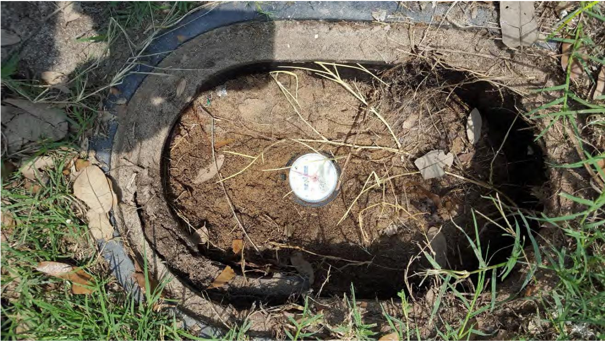
Photo 7 – Cycle 16 Meter at 168 Nueces Dr (excessive dirt/debris to be removed from meter box; replace meter box due to deteriorated condition):
